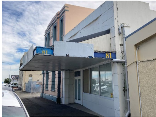
Deteriorating building. Childers Rd
