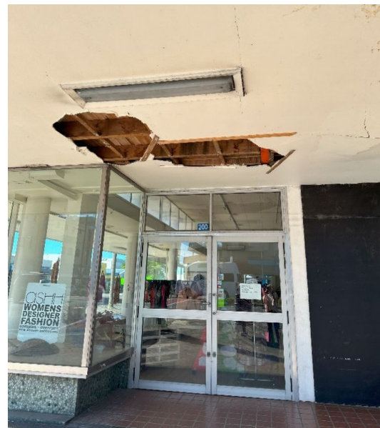
Main Street building decay. Gladstone Rd
