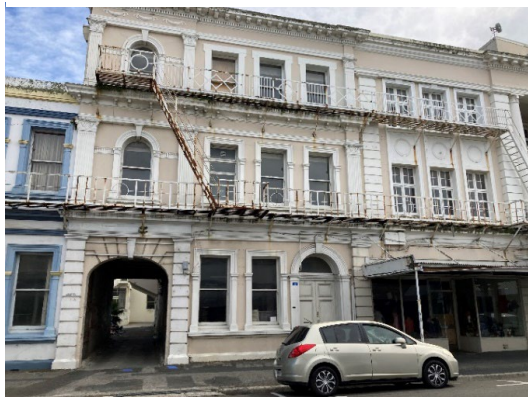
Masonic Hotel decaying façade. Lowe St
